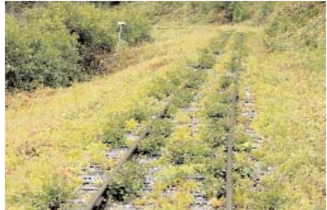
Overgrown weeds on the track bed are nearly impossible to get rid of with non-chemical methods.
