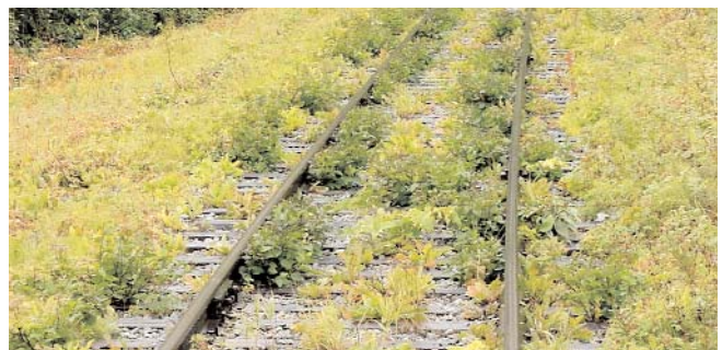
Overgrown weeds on the track bed are nearly impossible to get rid of with non-chemical methods.
