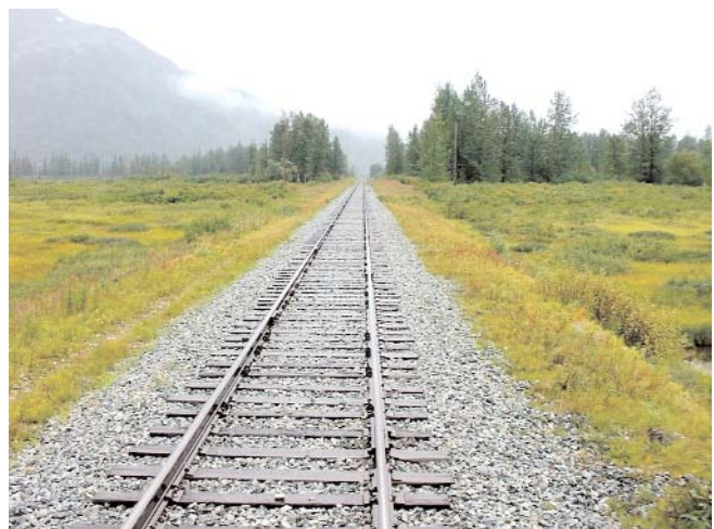
Optimally, the Alaska Railroad track would be free of weeds, providing an uncompromised platform for train movement.
