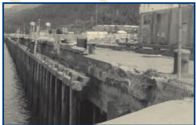
The Marginal Wharf was condemned in spring 2002 for safety reasons.
