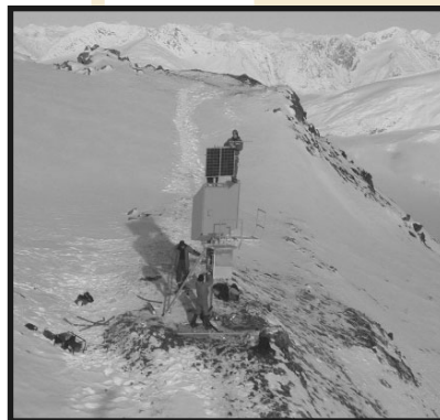
A blaster box is installed by an avalanche path near Girdwood.
