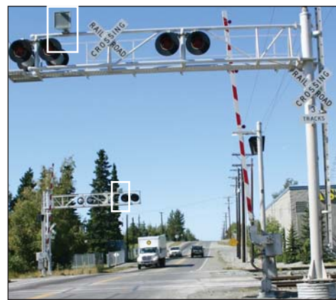
Automated wayside horns at Klatt Rd crossing.
