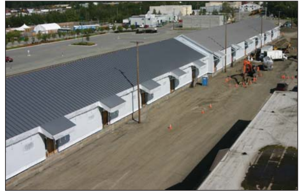
August 2009: After installing substantial insulation, contractors erect new siding on the front side of the shed.
