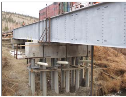
The old bridge MP 432.1 (above, top) was comprised of three open deck girder spans. It is being replaced (bottom) with two steel girder spans with concrete ballast deck tubs, and new piling with thermopiles to keep melting permafrost frozen (thermopiles are used on the Trans-Alaska pipeline).
