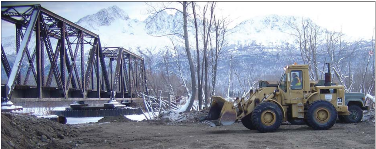
Work gets underway to rehabilitate the timber piers at Matanuska River Bridge (ARRC Milepost 148.3) .
